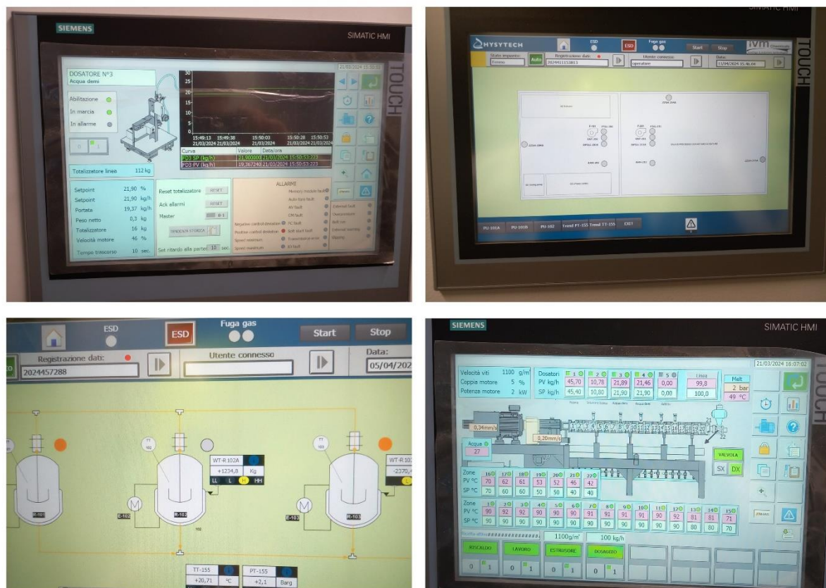
Figure7. Emulsification line control system examples
